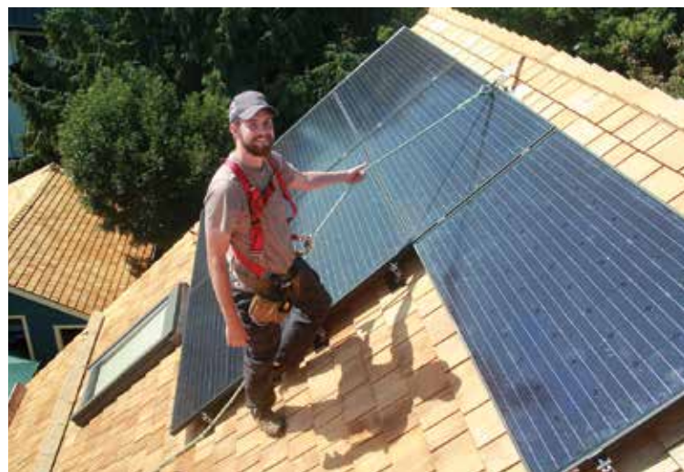
Electrical engineering co-op student Brian Vincer during an installation of solar panels in the Cook Street area.
